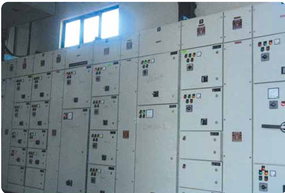
CONTROL PANEL FOR POWER PROJECTS
